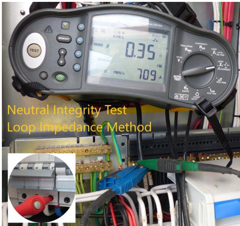
Figure 4 – Example of neutral integrity test.
